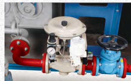
Steam Flow Control Valve
