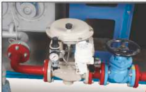
STEAM FLOW CONTROL VALVE
