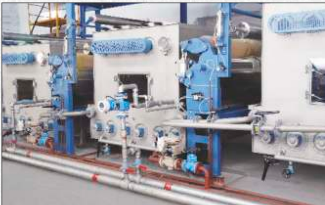
WASHING TANKS WITH VARIOUS CONTROLLERS
